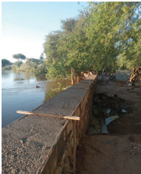
Figure 5.5: Flood retention walls upstream of Beledweyne (constructed by Hiran Development Program in collaboration with community-led initiatives)
